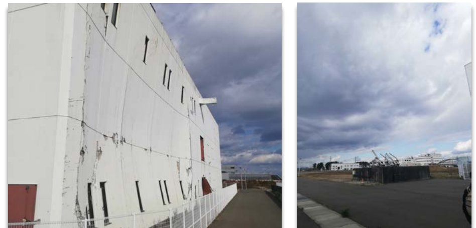
Figure 5: View of damaged parts of buildings and sections, at the Minami-Gamo Wastewater Treatment Plant, after the tsunami
