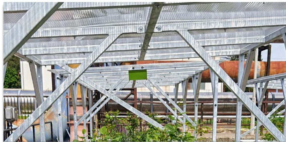
Technical facilities, first floor of the recovery plant © HAMBURG WASSER/Julia Unkel
